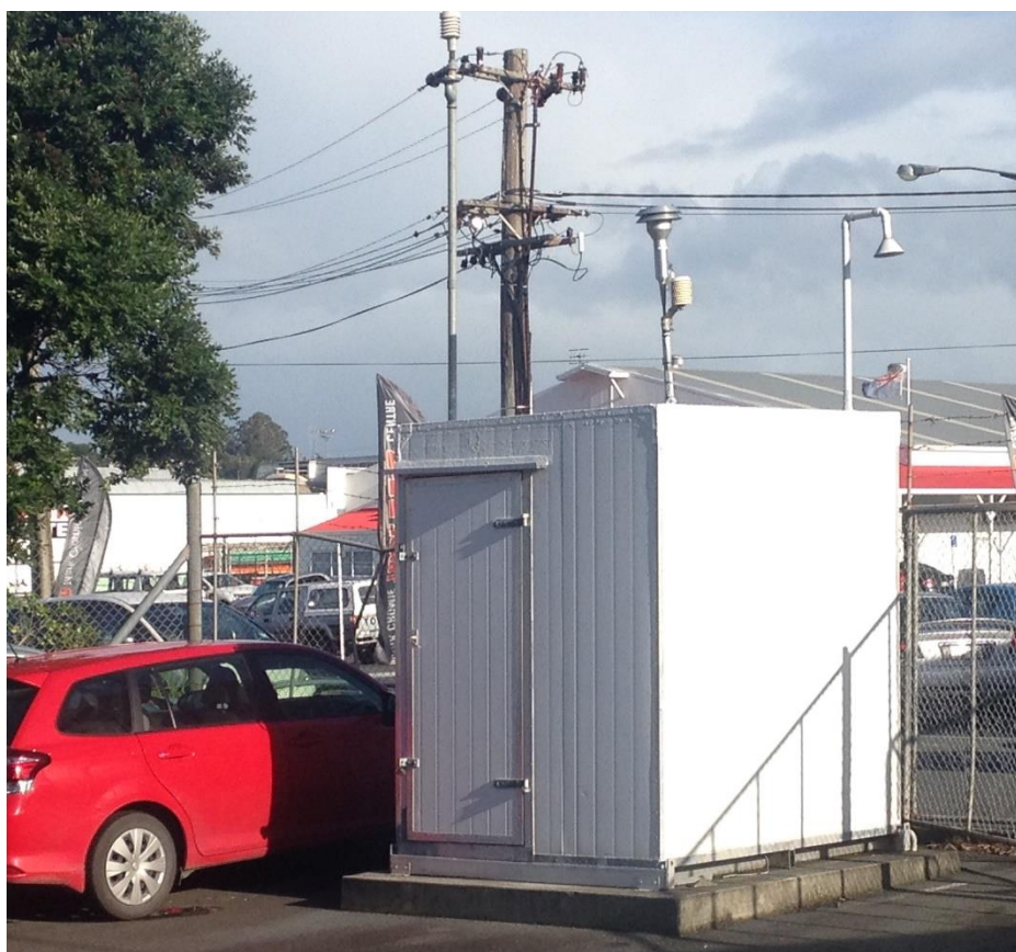
Air monitoring shed at Robert St, Whangārei
