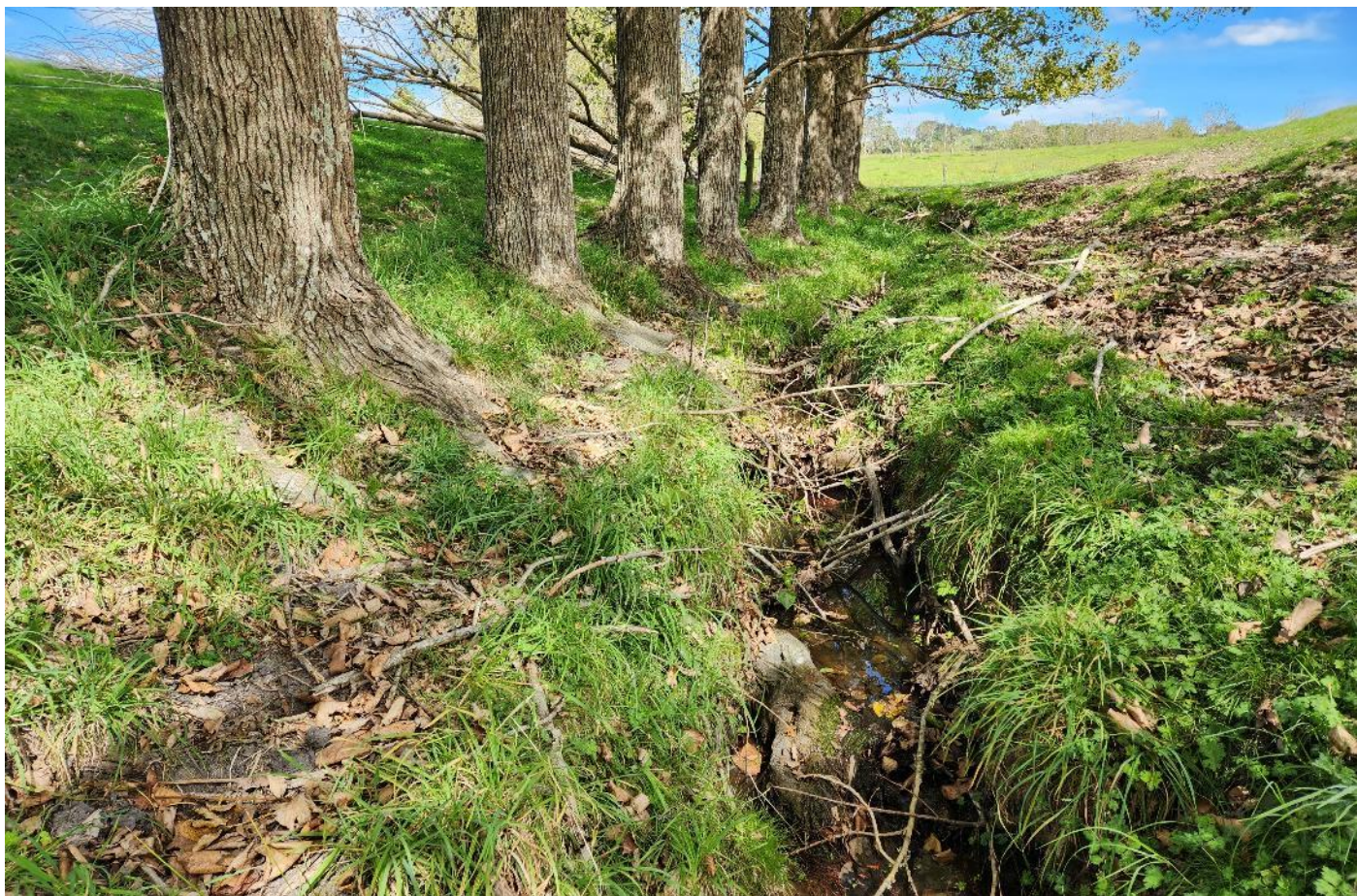
Kawa roots plunging underneath the drain. Set poplar back further to reduce risk of toppling.
