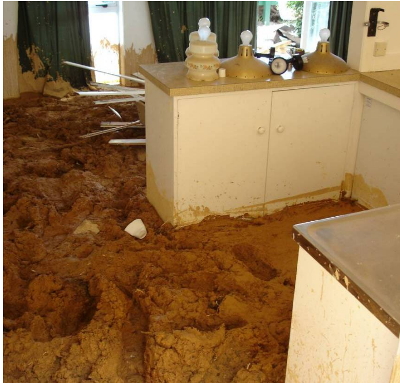
Figure 16: Mud on the carpets at Haruru Falls Resort.
